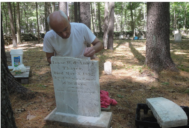
The bottom piece is level and has been set. Then epoxy is applied and the two pieces are joined. They are then clamped together
